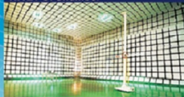
10m Standard Anechoic Chamber
