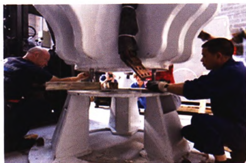
国外客户安装现场 Installation in the foreign customer's factory
